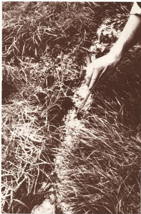
A poorly placed septic field in Wilton, Ct., near a steep slope and wetland, resulted in septic out-break, creating a surface health hazard and endangering the well of the adjacent residence.
