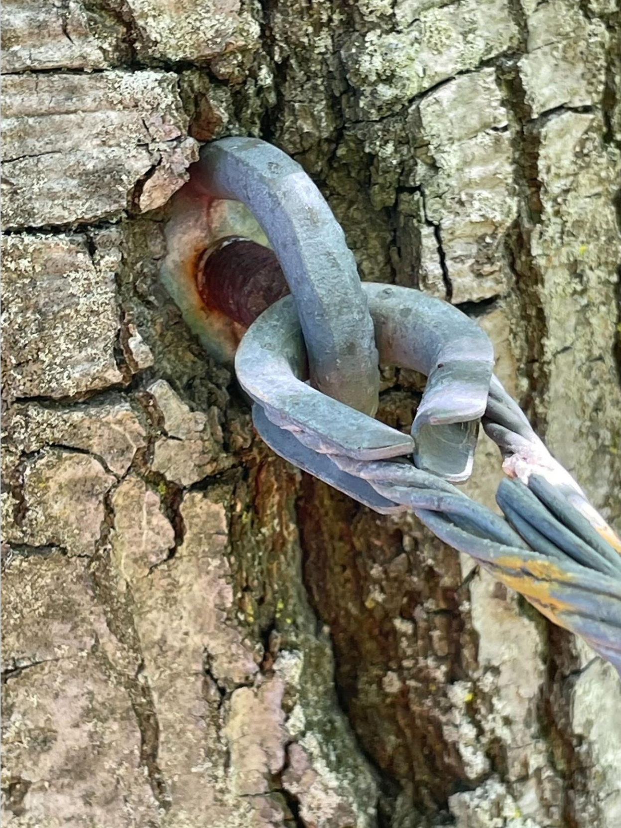
Image of a deformed 1/4" thimble installed in the crown of the tree.
