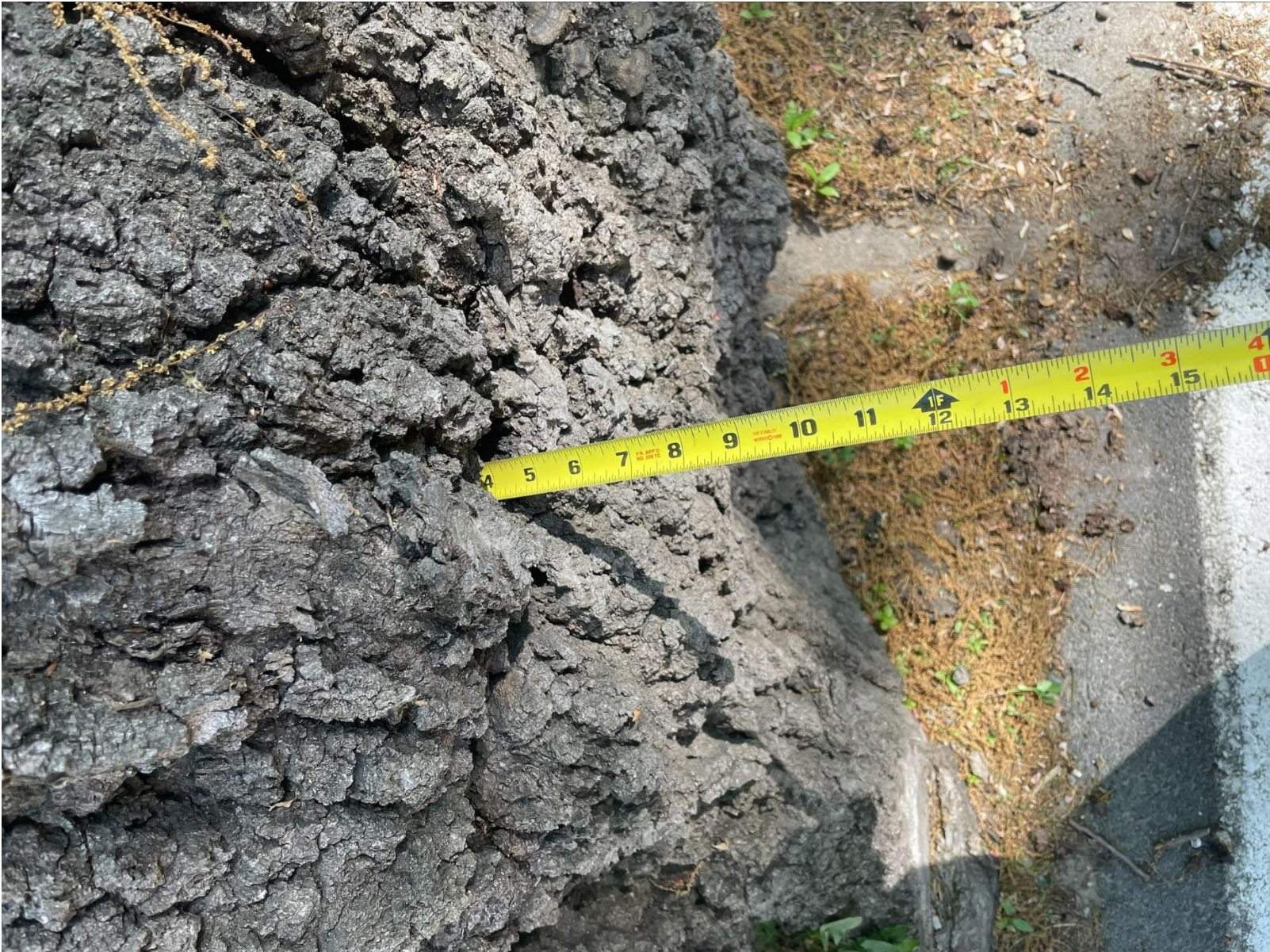
Image of depth of lateral crack.
